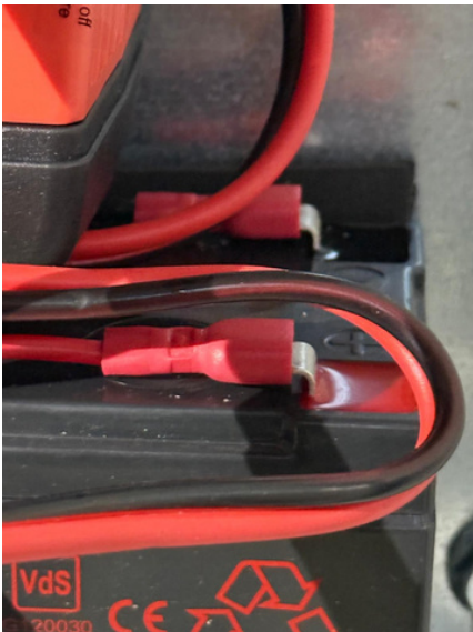
Battery terminal clamp.
